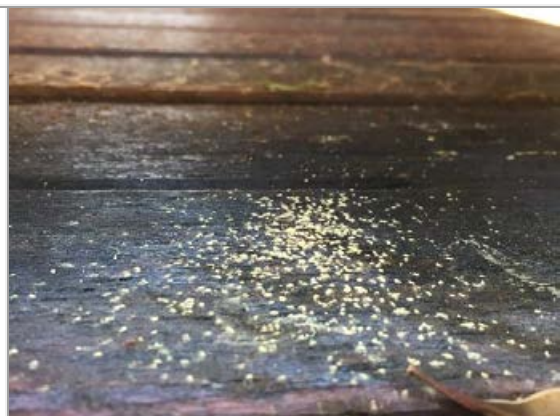
Frass on the deck under
