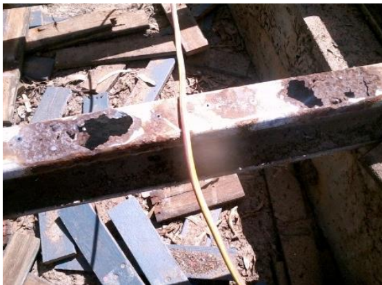
Badly rusted steel joist
