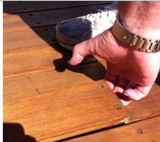
Broken screws in steel joists
