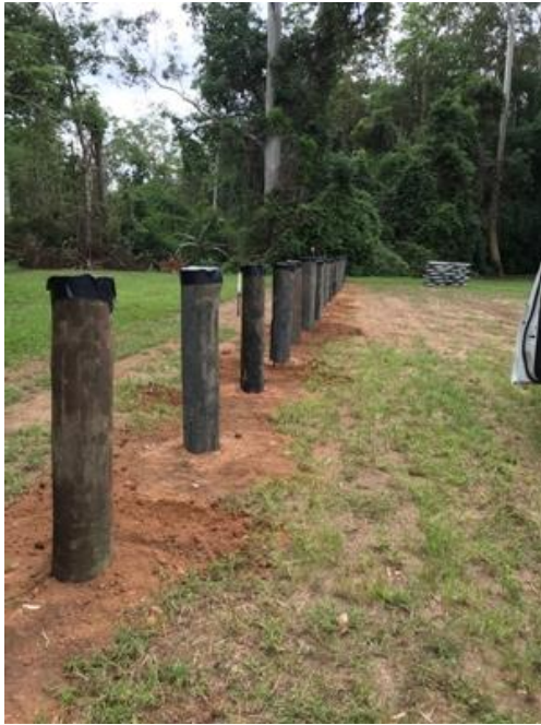
Figure 1. Poles in test at the new DAF Nambour test site
