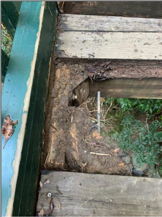
Decomposed leaf litter, moisture and dirt entrapped moisture accelerating decay effects
